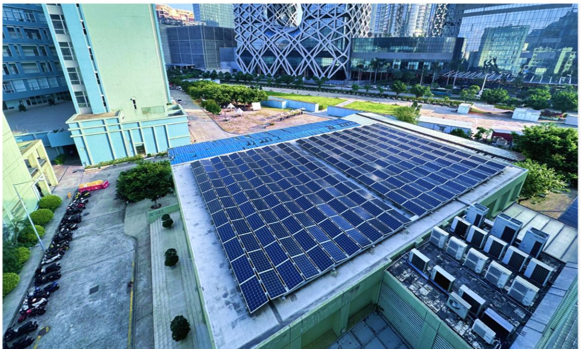
Fig. 14 Solar panels in Block D
